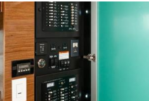
2013 Cruisers Yachts 45 Cantius - Main Distribution Panel
