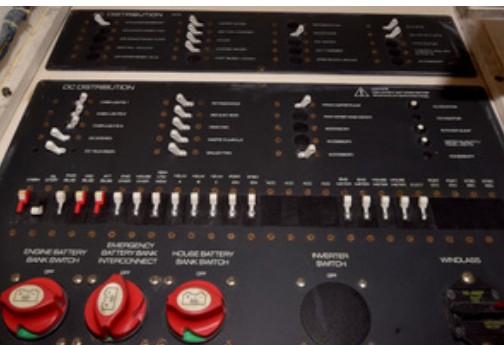
2009 Tiara 32 Open - Breaker Panel
