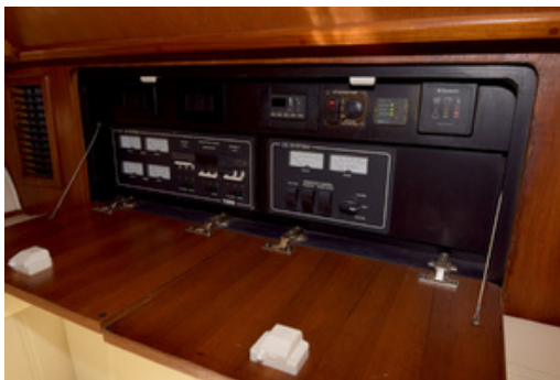
2009 Tiara 32 Open - Electrical Panel
