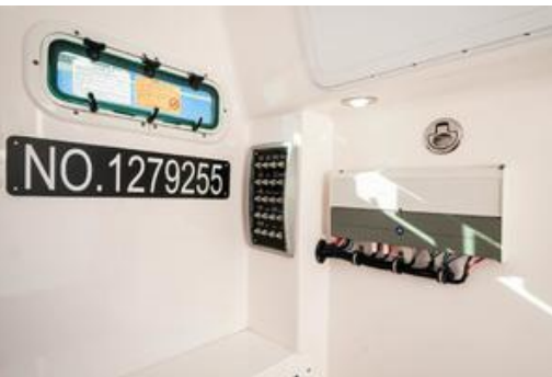
2015 Everglades 325CC Power Amp And Breakers
