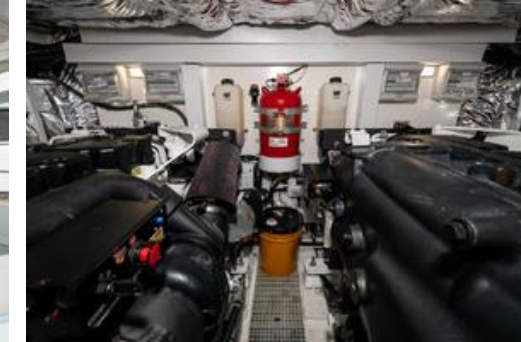
2016 60 Princess FB Engine Room (1)
