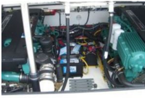
2005 Tiara 2900 Classic LE - Indeed - Engine Room
